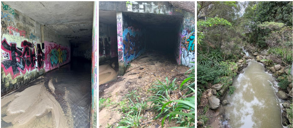
Figure 6. Opening into the daylighted section of Brookvale Creek along Old Pittwater Road (ID 2 Figure 4 ). From left to right: a) Functioning culvert. b) Sedimented deposition in the culvert. c) Rock-lined transition into the stabilised channel immediately downstream of the culvert.
